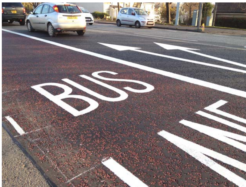
Glasgow Road - red chips embedded in HRA surface course
